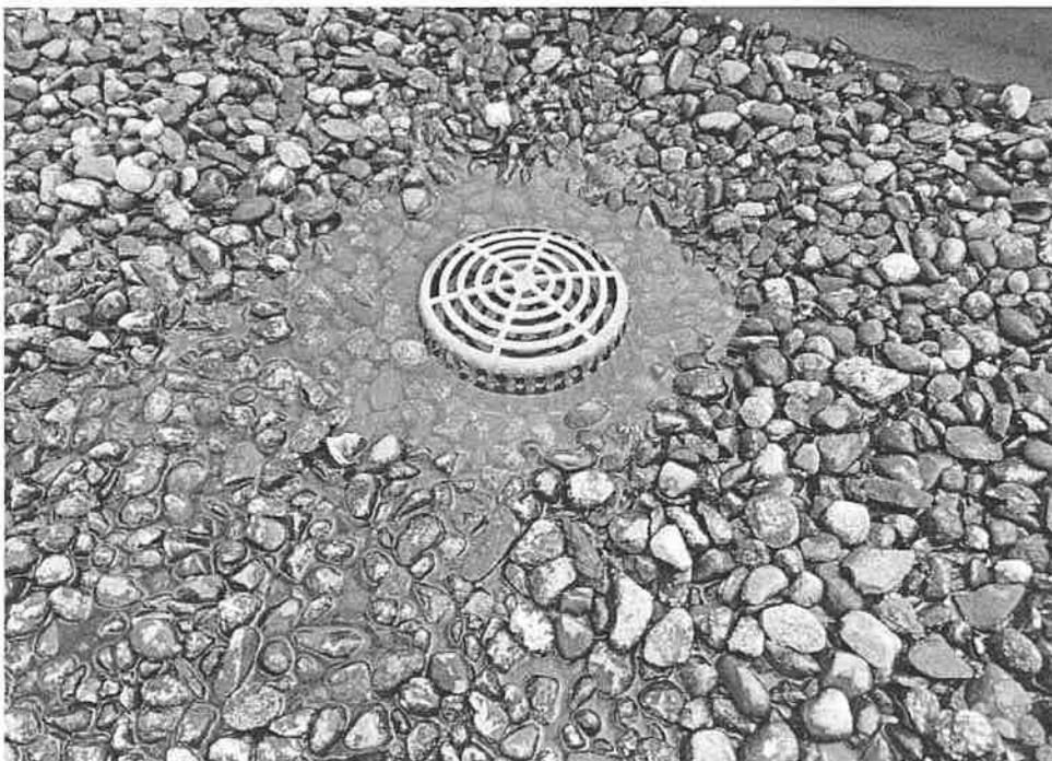
Drain clogged due to ballast and debris around it.
