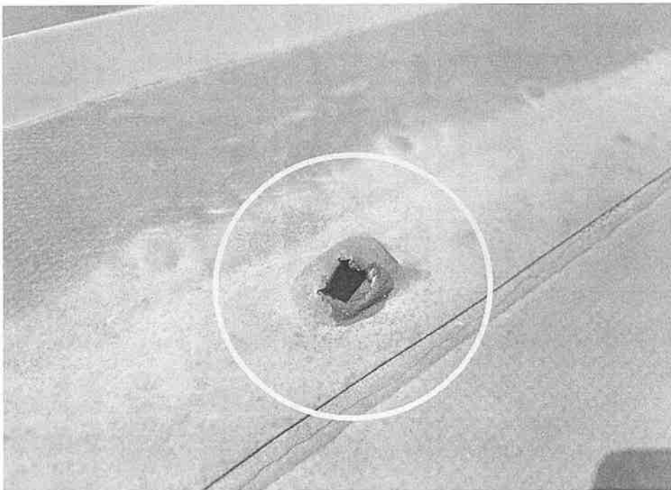
Open condition around perimeter EPDM membrane – could cause water intrusion within the insulation.
