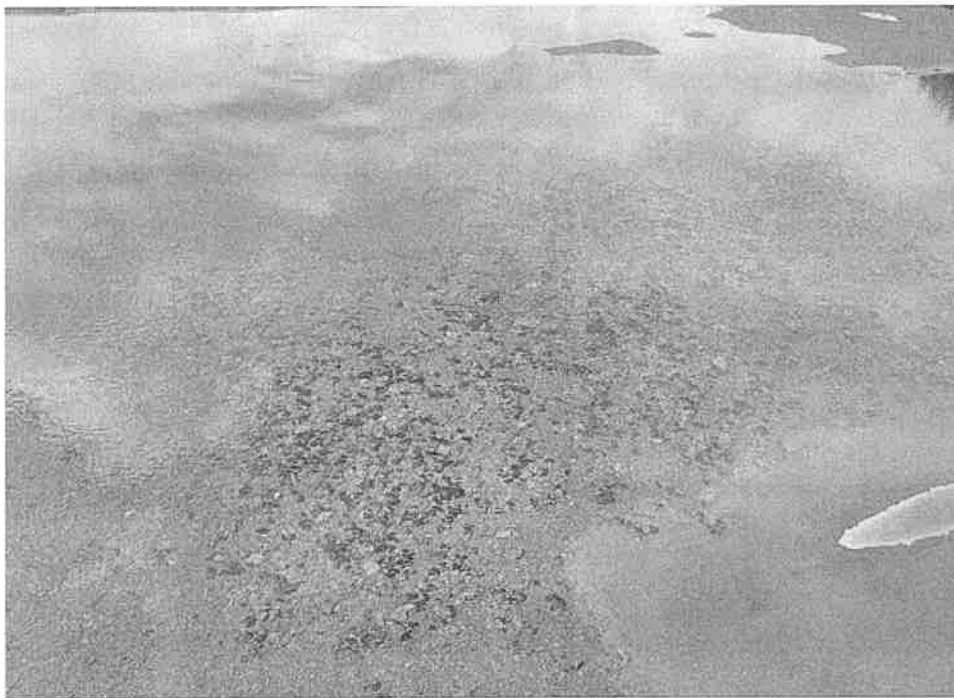
Ponding present throughout the roof. Ponding occurs when there is a lack of pitch and the water pools.
